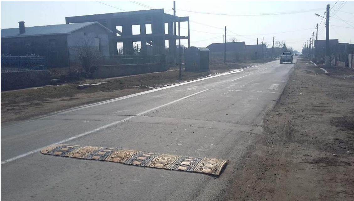
Figure 12 – DJ226 Road conditions in Corbu
