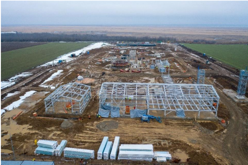
Picture 3 and 4 Gas Treatment Plant in Vadu
